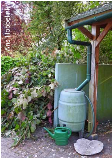
This shelter is used to collect rainwater.
